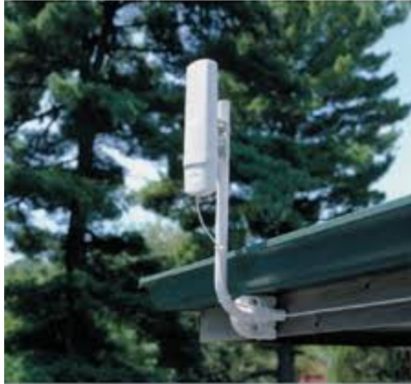
Eave mounted Radio and Mounting
